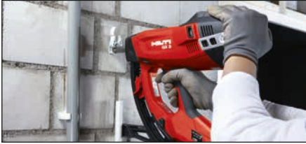
Conduits and light-duty pipes
